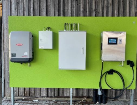
1 DC Ladestation 22 kW
